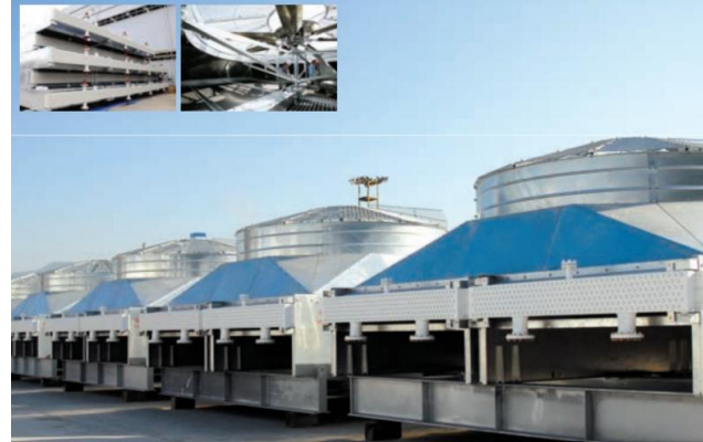
Air Cooled Heat Exchanger
